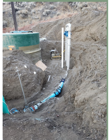
Chamber and piping
